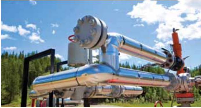
A natural gas well in Alberta.
